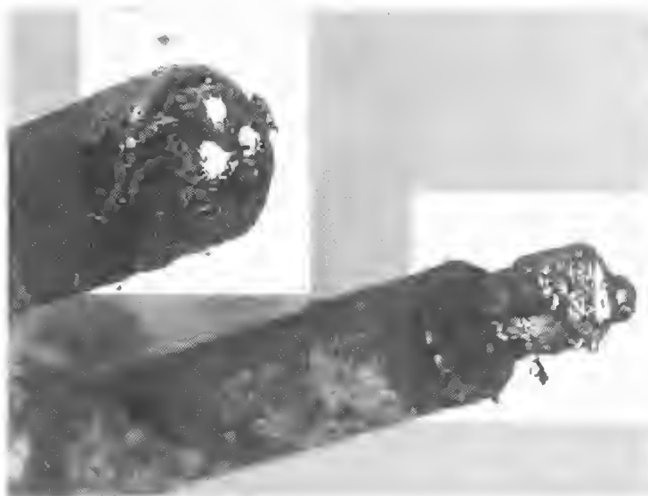
FIG. 9. A computer-enhanced photograph, taken from an original held by SEQEB, of the remains of both the two-core and the three-core systems emerging from the wall of the cellar of Parliament House (cf. Fig. 8). These were destroyed during the 1980s renovations of this building.
